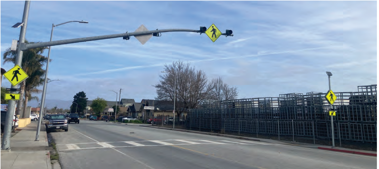
Rectangular Rapid Flashing Beacon in Pajaro.
